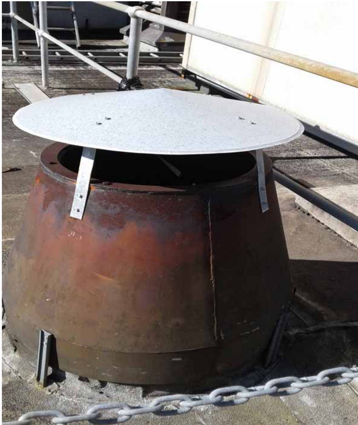
Photo 12 – View of toilet exhauster
