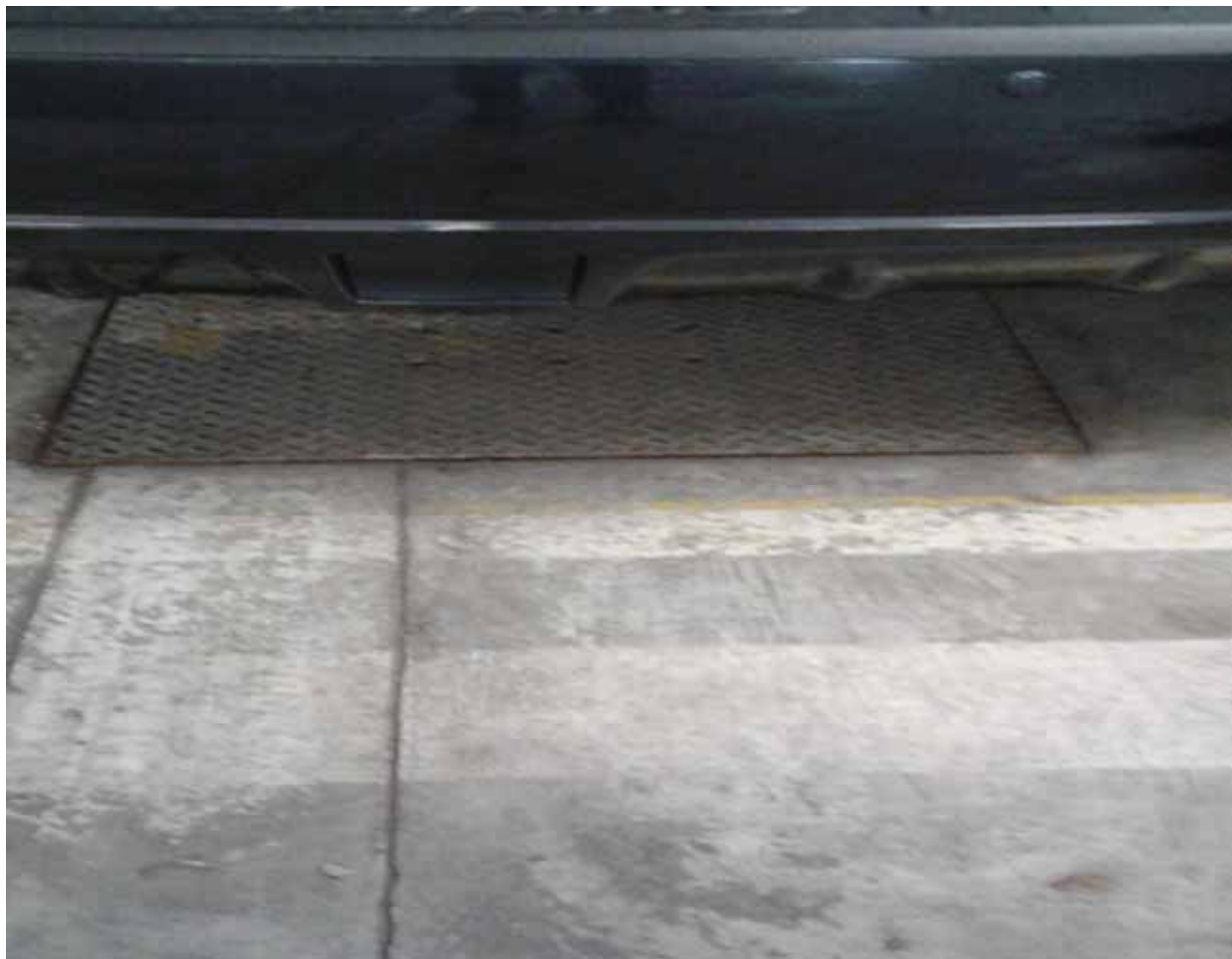
Photo 17 – View of underground fuel tank
