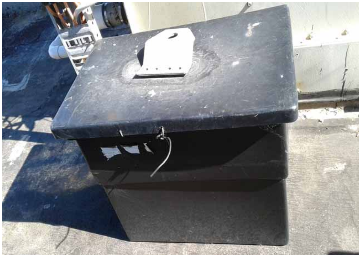
Photo 11 – View of coolant chemical storage
